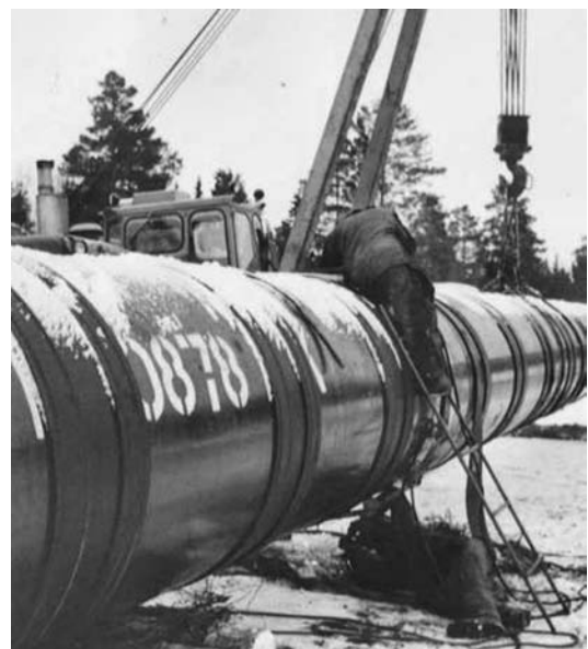
Figure 2: A pipeline-welding site in Russia where LB-52U is used for joining the girth joints in freezing weather.
